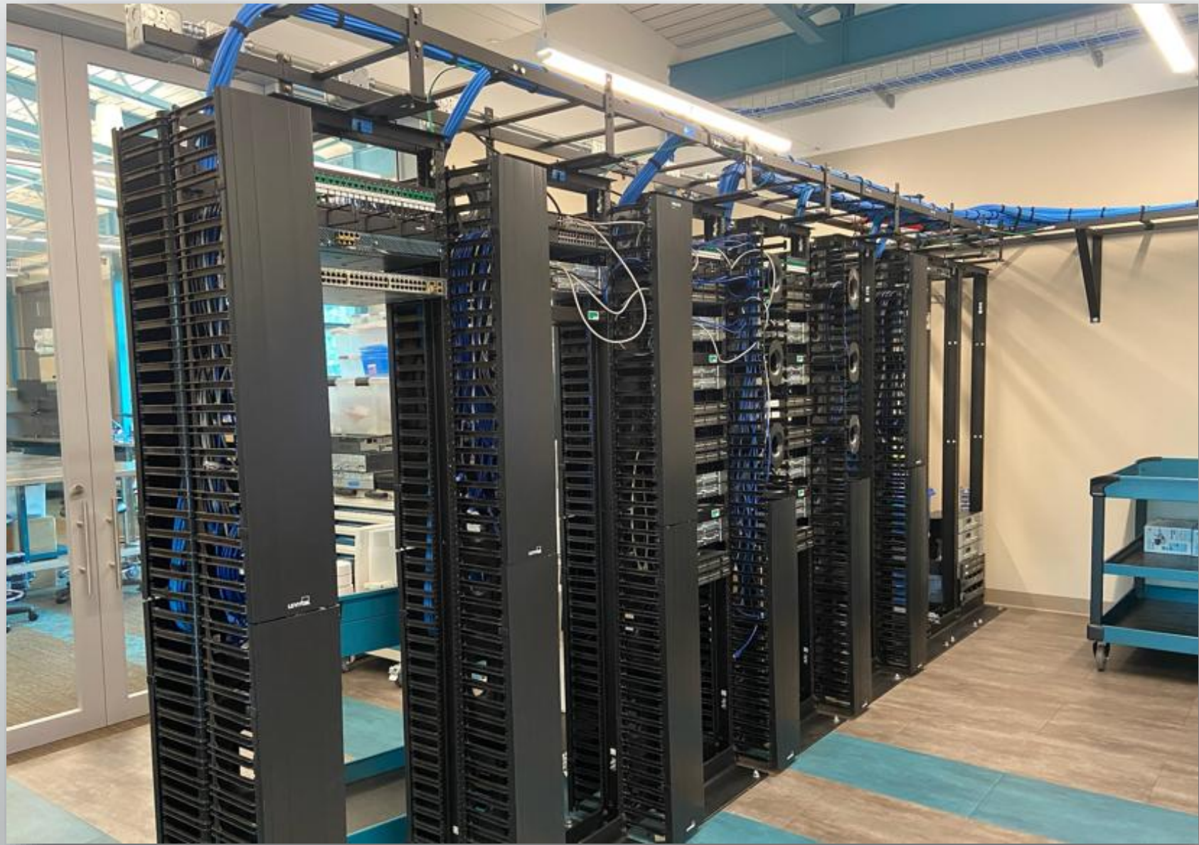
CIS Building Data Center
