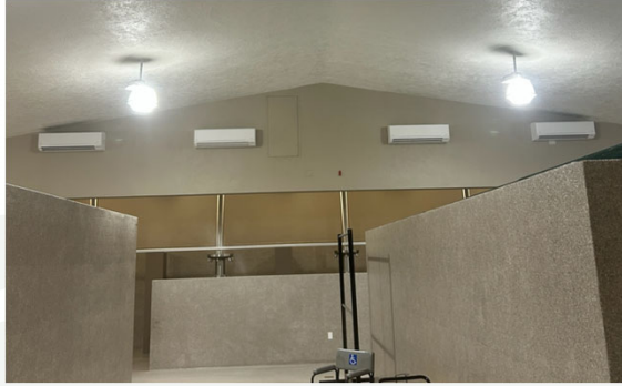
Locker Rooms HVAC
