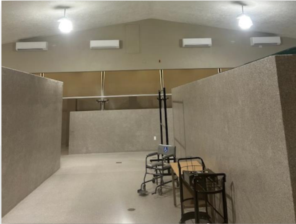
Locker Rooms AC
